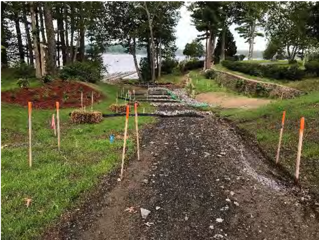
Fig 4: Temporary BMPs on slope above manhole at Gundalow Landing/east side of the bay. View southwest. (07-20-20).
