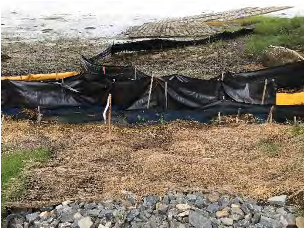
Fig 6: Temporary BMPs on toe of slope below manhole at Gundalow Landing/east side of the bay. Viewing southwest. (07-20-20).
