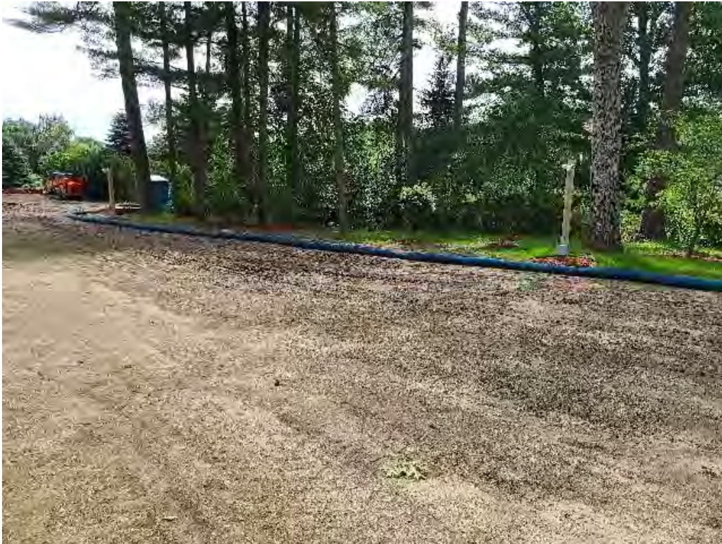
Fig 1: Filter sock at Gundalow Landing/east side of bay to prevent potential sediment-laden water from exiting the site. Viewing southeast. (07-16-20).
