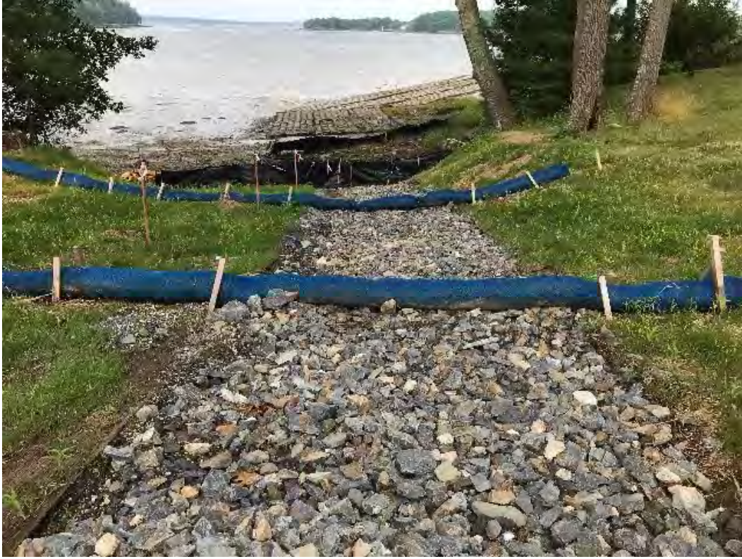
Fig 5: Temporary BMPs on slope below manhole at Gundalow Landing/east side of the bay. Viewing southwest. (07-20-20).
